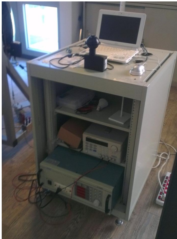
Fig 2. Electronic control (DC, AC and Ballast control units)
